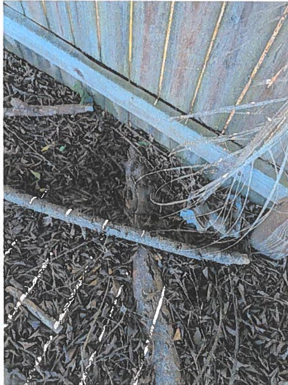
These large roots are causing damage.
